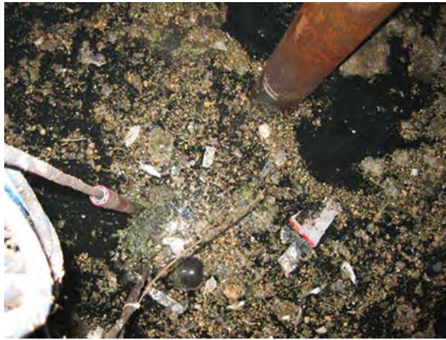
Figure 5-5: Existing reclaimed water wet well (photo by Terry Mitchell, 2011).
